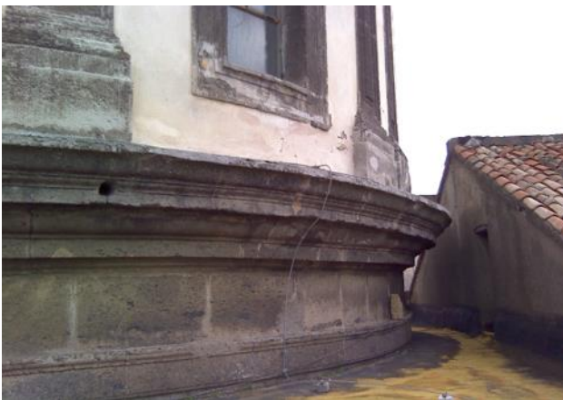
Figures 11 and 12. Santa Caterina a Formiello Church. The elevation of the drum and, below, detail of the cornice in Piperno stone at the base (photo M. Facchini, DiARC MLab, 2019).
