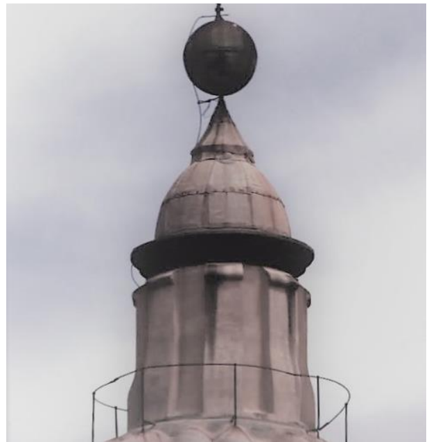
Figure 14. Santa Caterina a Formiello Church. The brick lantern rebuilt after the earthquake of 1688.
