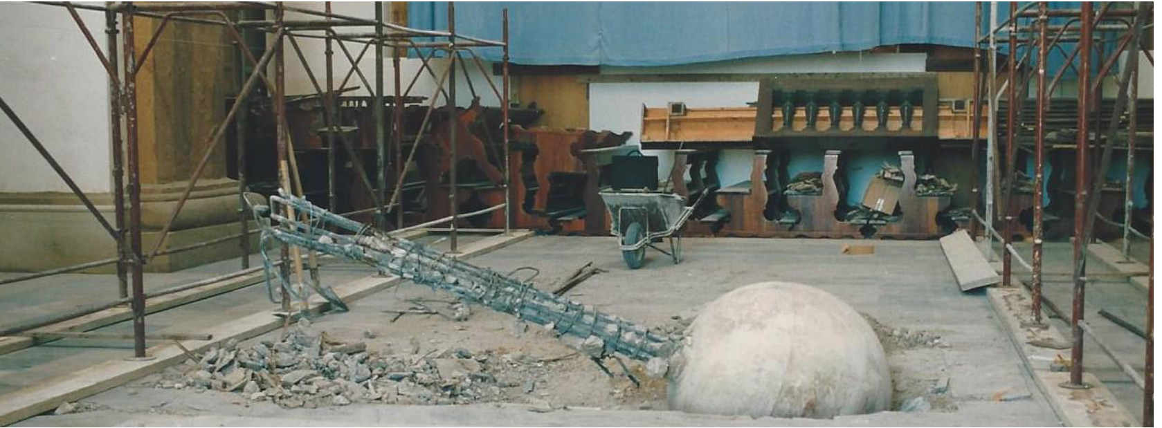
Fig. 8-10: Disconnection of the masonry following the detachment of the sphere; Hole in the cover caused by detachment and falling of the sphere; Stone globe with cross in the central nave after falling from the bell tower [Berenato 1994].
